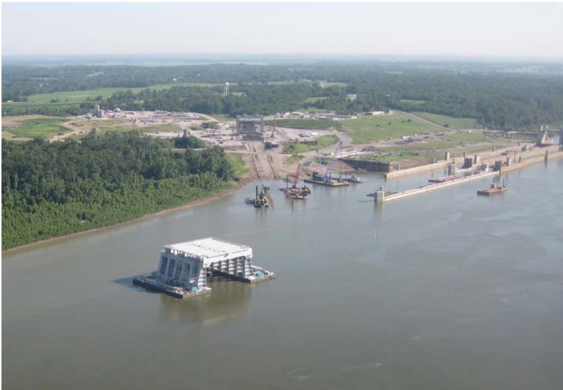
Pictured is the 5000-ton catamaran lift barge. Due to bridge clearances, final assembly is done on site. In the background, the casting yard, launch ways, and shore side travelling lift for the shells are being constructed. (Washington Group/Alberici Photo)
