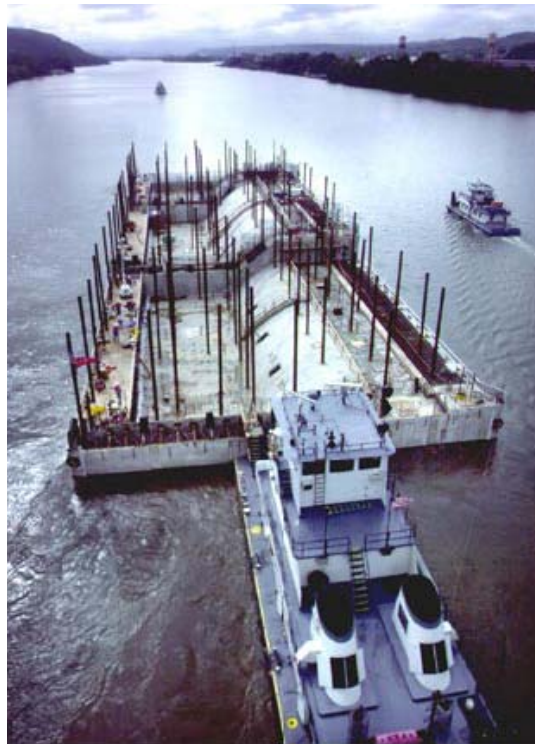
Braddock Dam Shell Segment 1 being delivered down the Monongahela River. At this time, the grout and tremie injection pipes were already installed.
