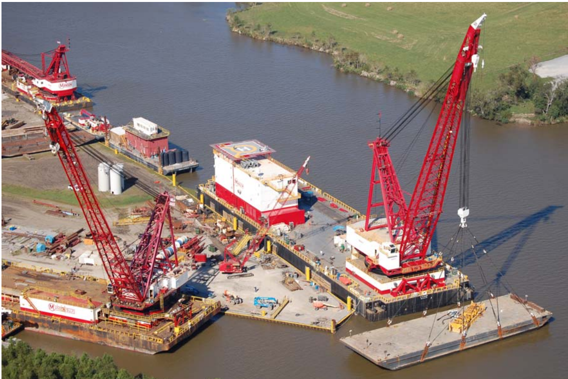
Shown is the 1100 short ton proof load test using a water-filled barge. The testing was performed at Manson's Houma, Louisiana facility. (Manson photo.)
