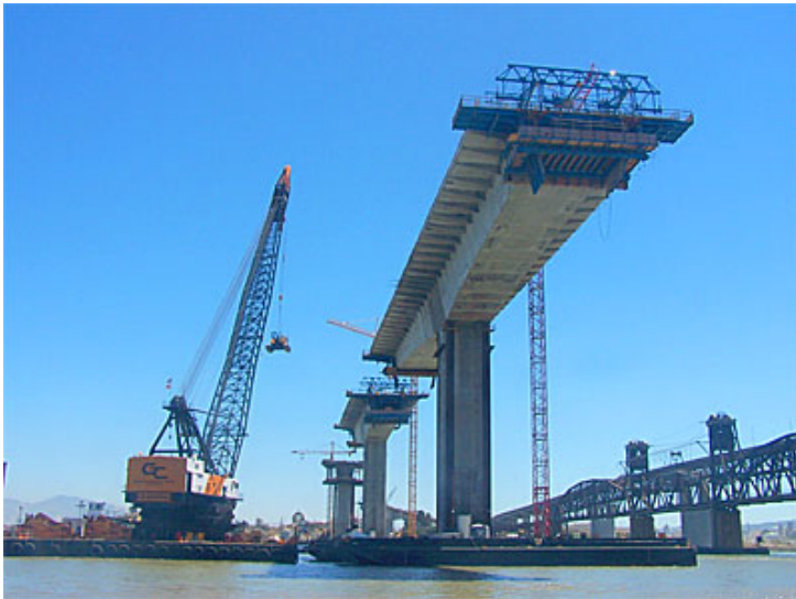
Shown left is the D.B. General at work on the Benecia Bridge across the Carquinez Strait.
