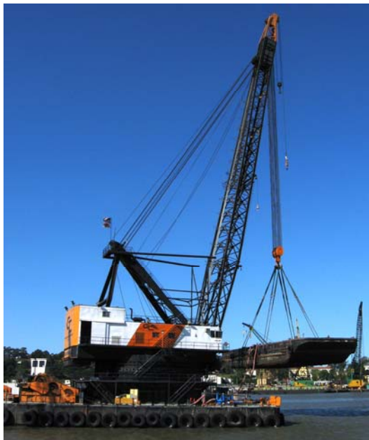
Shown left is the lift of a water-filled barge for the 770-ton proof load test..
