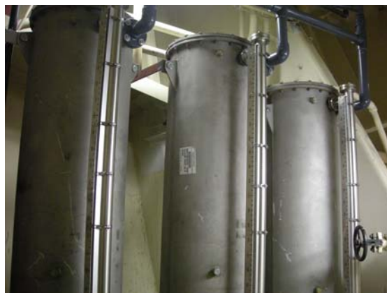
Figure 9. Sodium bisulfite tanks located in engine room.
