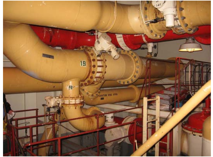
Figure 3. Ballast water discharge line in the pump room.
