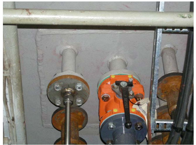
Figure 5. Bisulfite and hypochlorite penetrations of the engine room bulkhead.
