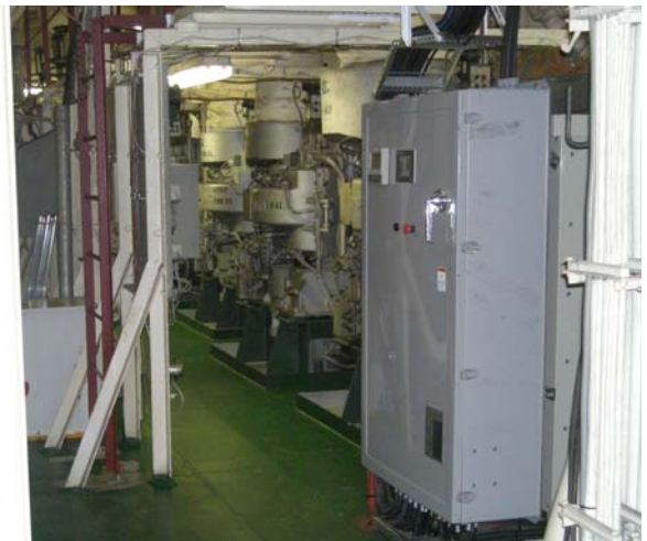
Figure 2. Main Control Panel for Hypochlorite Generator
